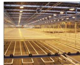
under bench heating
